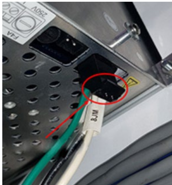
Figure 8-5 - Power to the Controller
